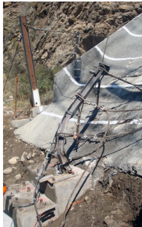
Upper left: CDOT's experimental runway. Lower left: Close up of the weld under attack.
